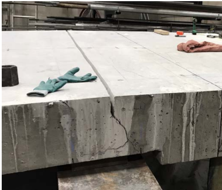
Figure 2-34. Saw cut at top of approach slab through top reinforcing for preparation of Test 2.
