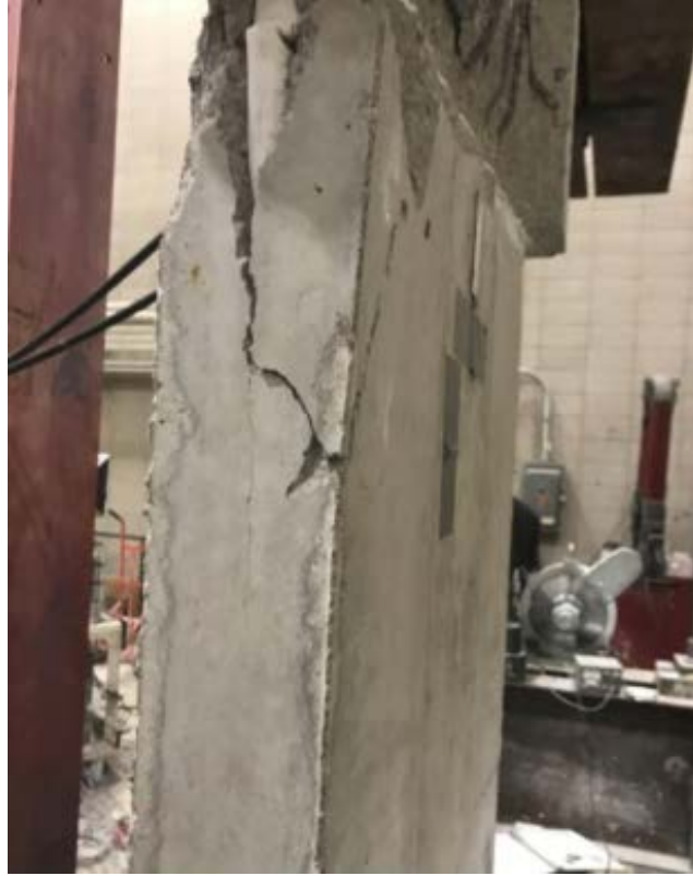
Figure 3-9. Crack developed within wall from bursting of top reinforcing concrete block.
