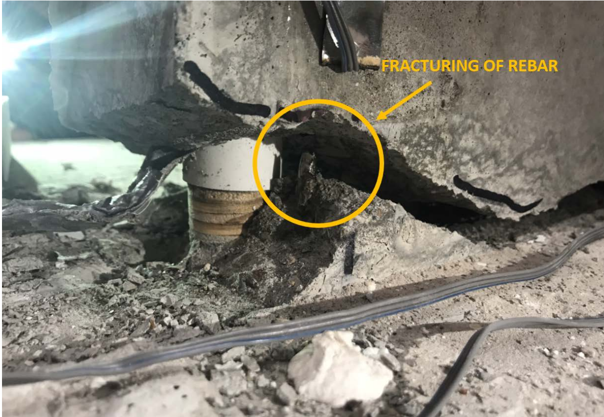
Figure 3-30. Fracturing of longitudinal reinforcing, pushover test.
